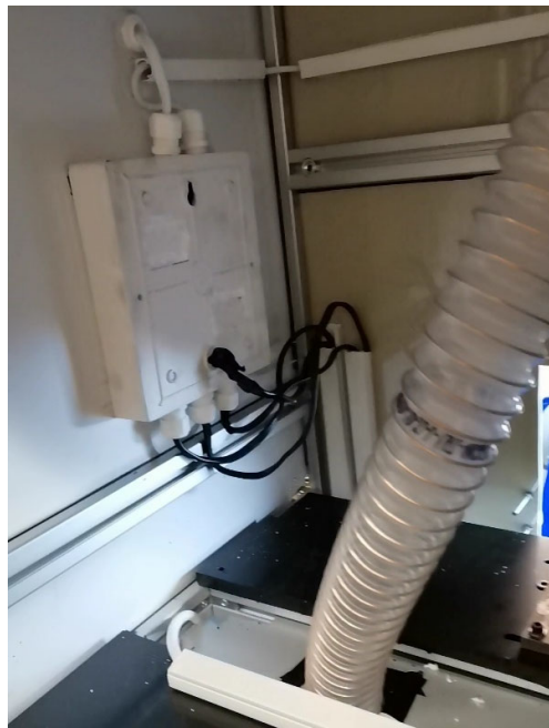
Figure A17 - Internal Distribution Board
